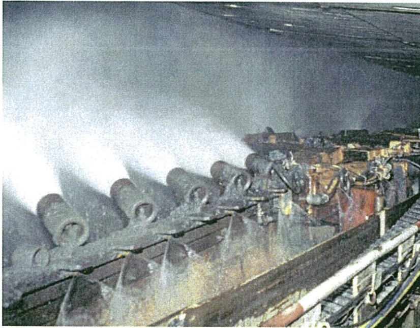
Venturi sprays mounted on headgate splitter arm.
