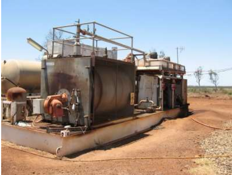
Figure 24: Tomlinson Boiler at an Australian coal mine (Zipf et al., 2007).
