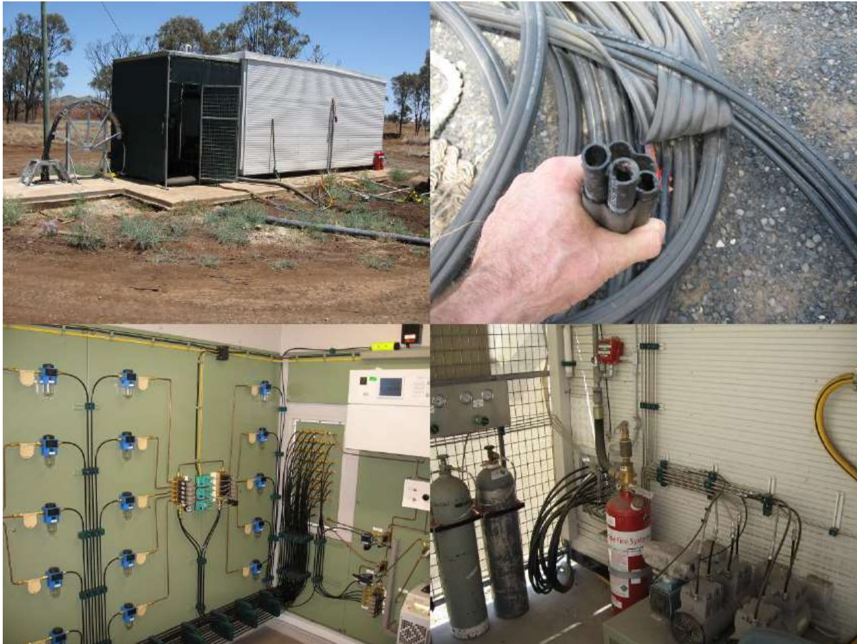
Figure 23: Continuous atmospheric gas monitoring system in Australia (Zipf et al. 2007). Top Left: Monitoring shed over mine showing borehole and sample tubes. Top Right: Clop-up of sample tube bundle. Bottom Right: Vacuum pumps. Bottom Left: Inside monitoring shed showing manifold system and gas analyzer.
